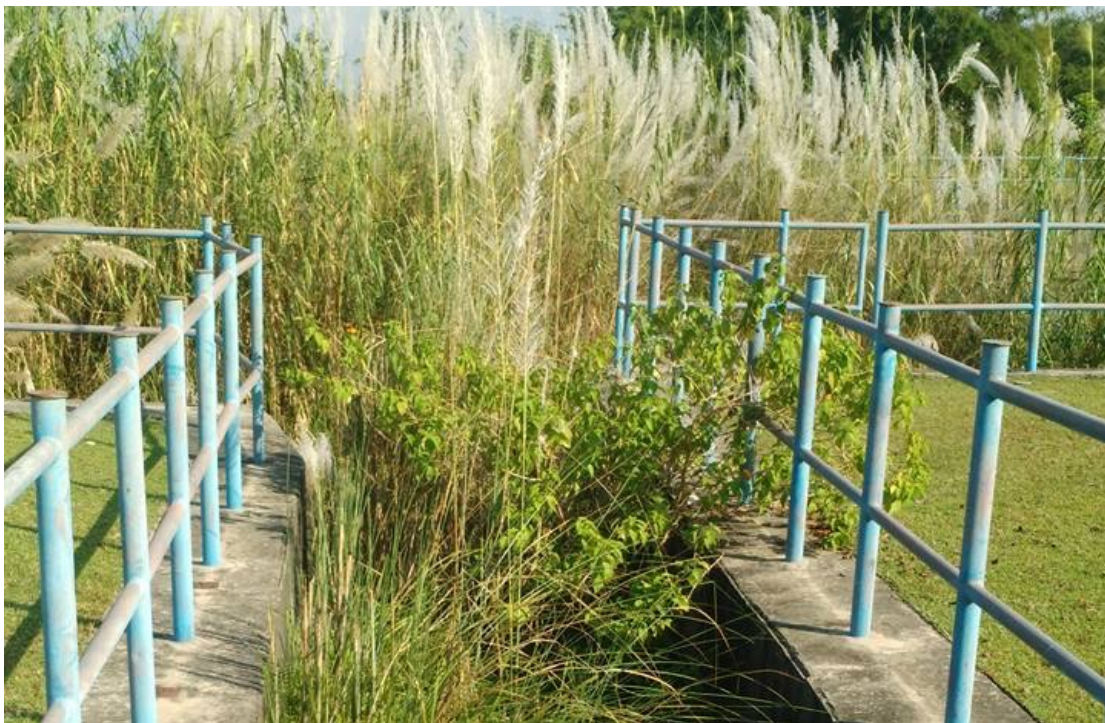
Figure 14. Example of one of the intakes to a secondary branch canal that was built in concrete as part of the RIP, but was abandoned within the first year of use due to rapid sedimentation.
