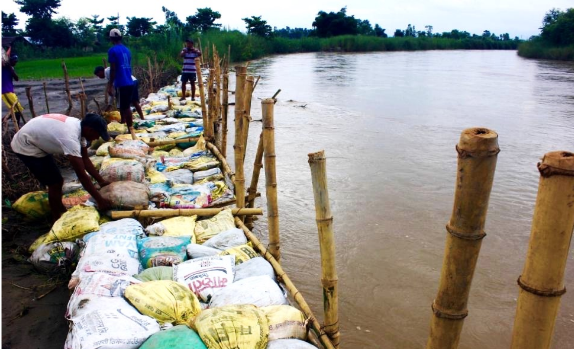
Figure 12. Farmers labor to construct an emergency structure to hold back the rising waters of the Budhi Kulo which threatens to overflow its banks and carry sand into their fields.
