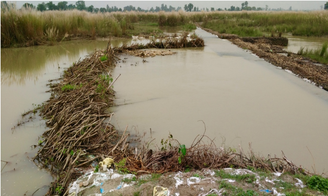
Figure 19. Here it is possible to see the wave-like structure of the Tharu dam used to reinforce the compromised concrete and gabion dams further downstream at the Kairichandanpur intake.
