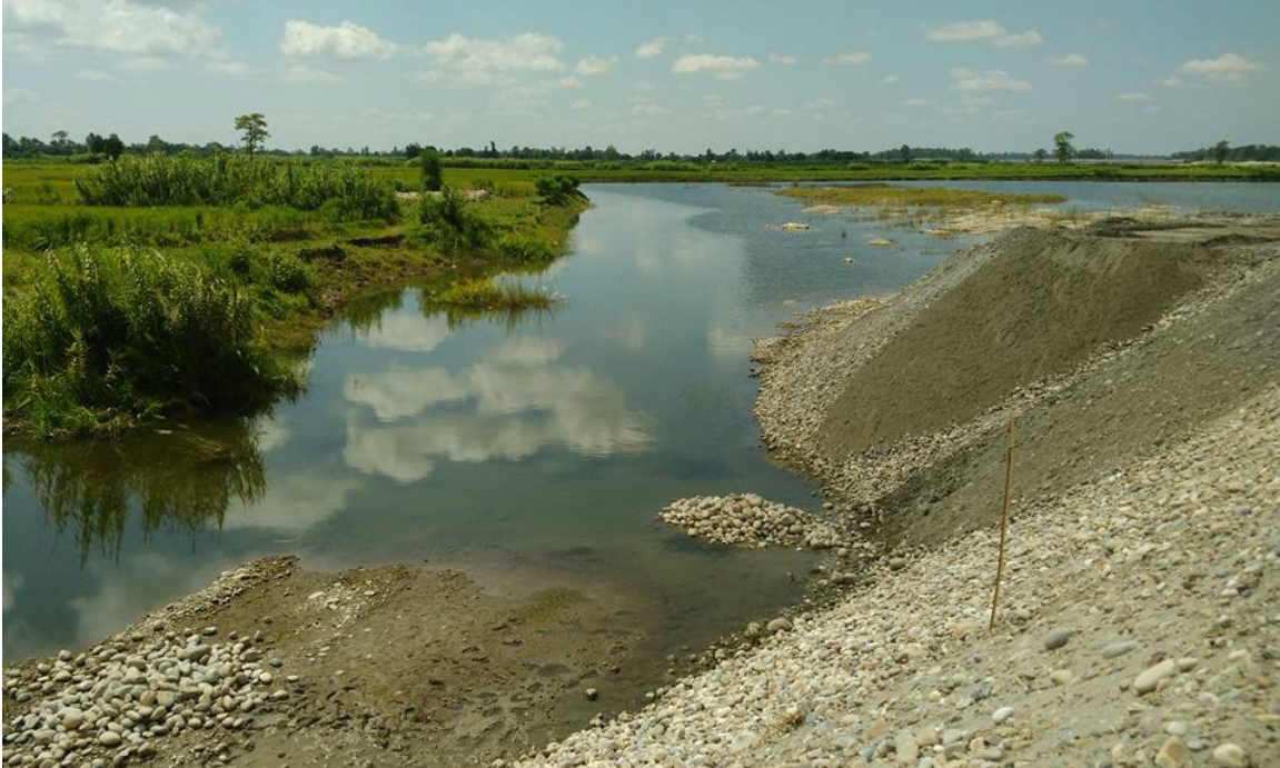
Figure 29. The waterlogged area on the left of this image is land that had been eroded by the Karnali River during the 2014 flood and that is being ‘reclaimed’ by constructing an embankment through the river.
