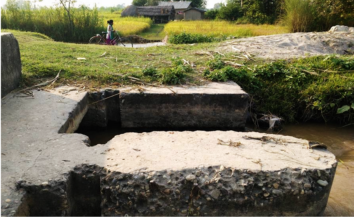
Figure 17. Concrete structure with scars where farmers used hammers and chisels to expand its opening.
