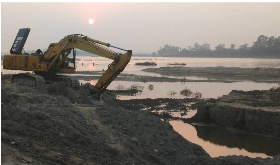
Figure 28. Excavator at an active construction site of the Karnali River Training Project.
