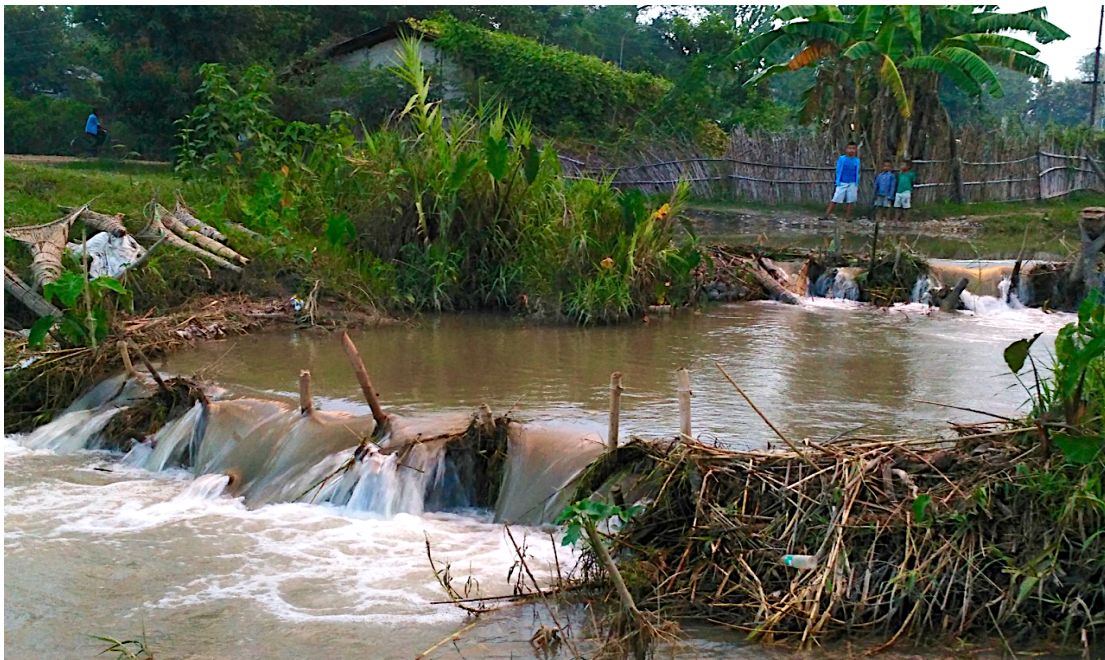
Figure 7. A series of farmer-built bandh whuas on a secondary irrigation canal in Rajapur. These structures are deconstructed and (re)assembled as necessary to direct the precise volume of water needed by farmers in smaller branch canals.
