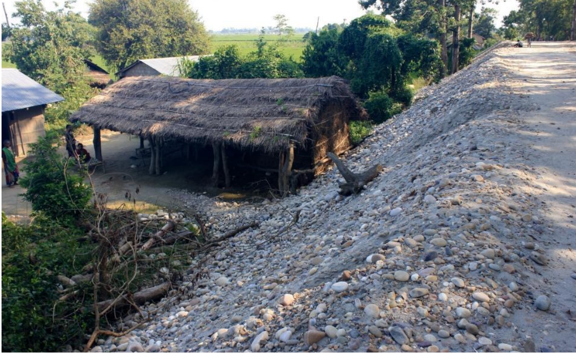
Figure 31. A partially-completed embankment built to ‘protect’ this community was not only built on their land, but has also created everyday challenges for them including waterlogging in their fields, erosion of stone and sand that washes into their yards, and difficulties in accessing the road and river.
