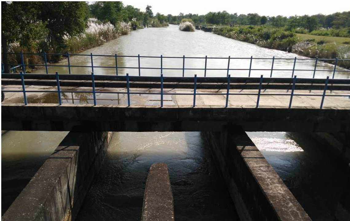
Figure 10. Concrete intake for the Budhi Kulo built at the northern reaches of the island’s farmer-managed irrigation system as part of the Rajapur Irrigation Project.
