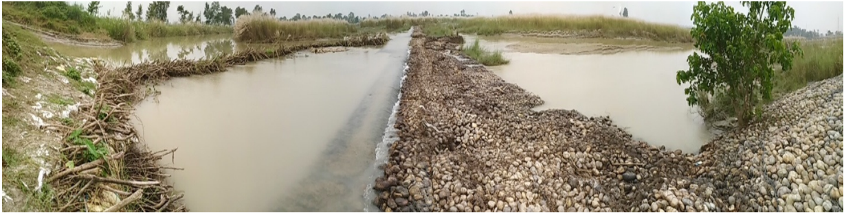
Figure 6. Layered dams on an irrigation canal intake, with gabion and concrete structures built by engineers as part of the Rajapur Irrigation Project and later reinforced using traditional Tharu technologies.
