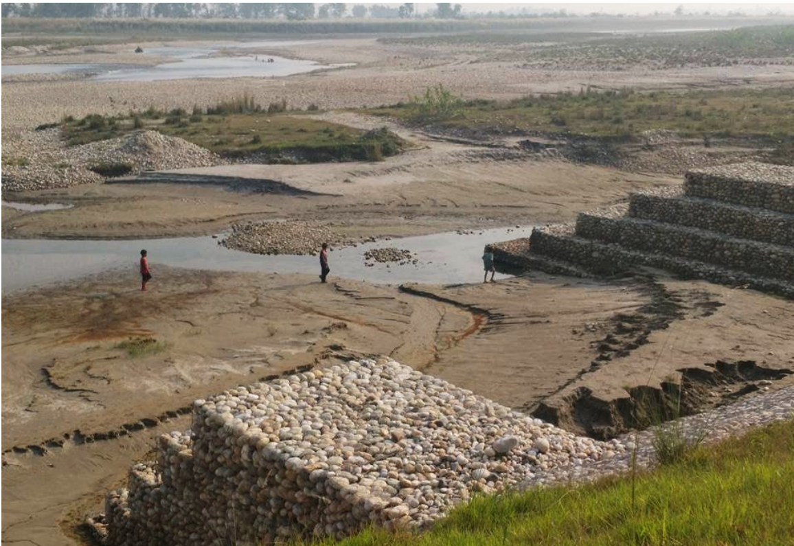
Figure 24. Embankment built as part of the Karnali River Training Project on the east branch of the Karnali River (also known as the Geruwa River). Here it is possible to see how embankments work to exacerbate sedimentation between spurs and deflect the river away from the 'protected' bank.
